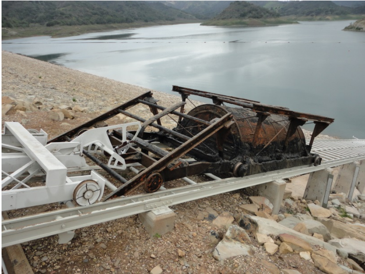
INTAKE SCREEN ASSEMBLY (screen and articulating cart)
