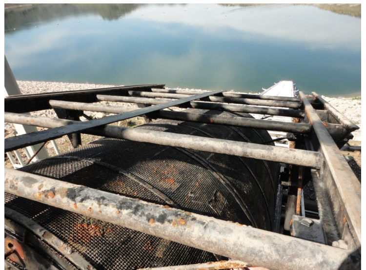
INTAKE SCREEN (topside view)
