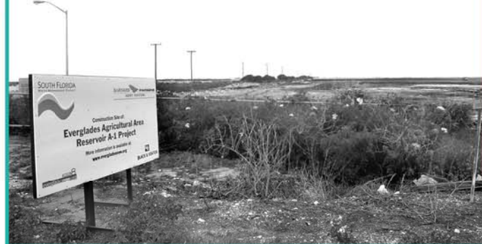
Construction is already underway for the South Florida Water Management District's "EAA-A1 Reservoir" Acceler8 project. The construction project is west of US 27, south of Belle Glade.
